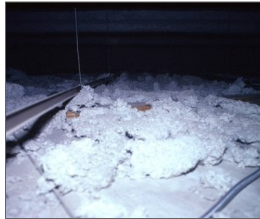
Debris from fireproofing on top of ceiling
