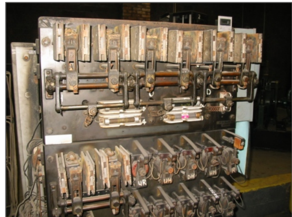
Transite Blocks in Elevator Switchgear
