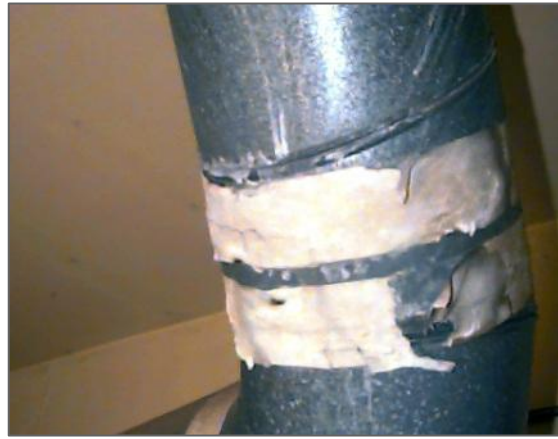
Paper on seams of duct
