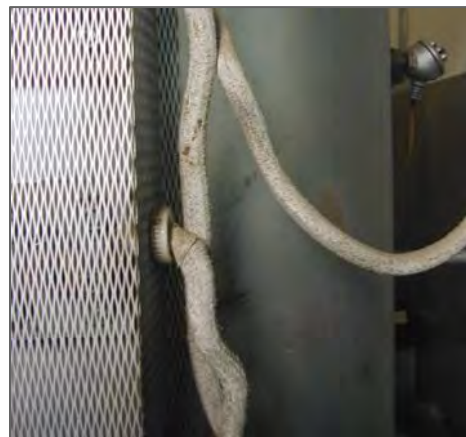
High Voltage cable insulation
