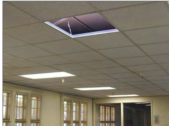
Lay-in ceiling tile
