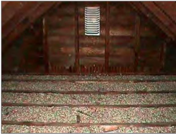
Vermiculite attic insulation
