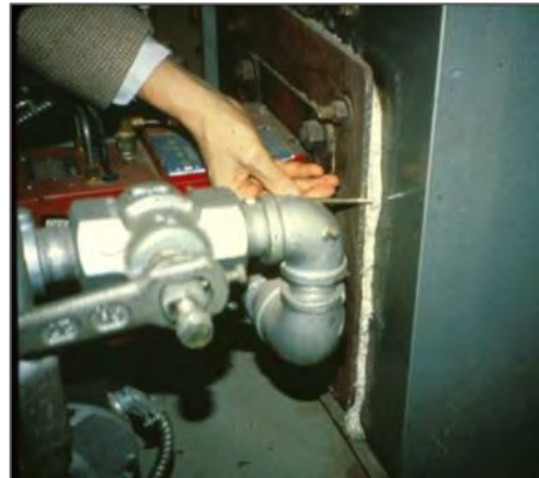
Rope gasket at boiler plate
