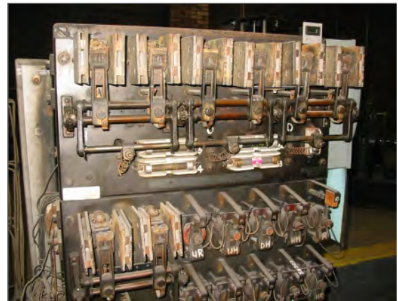
Transite Blocks in Elevator Switchgear
