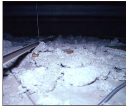
Debris from fireproofing on top of ceiling
