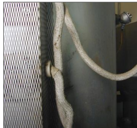
High Voltage cable insulation
