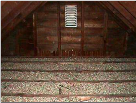
Vermiculite attic insulation
