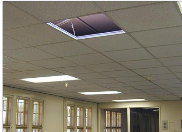
Lay-in ceiling tile
